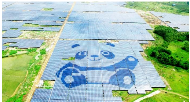
Guigang PV Power Plant in Guangxi Zhuang Autonomous Region
