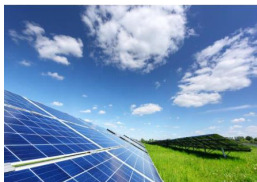
Guangxi Tianlin 120MW Agricultural Photovoltaic Complementary Project
