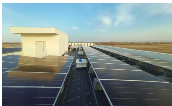
PV Energy Storage System installed on the rooftop of Datong Panda PV Power Plant
